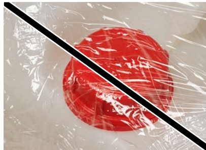
Venting holes blocked by foil
