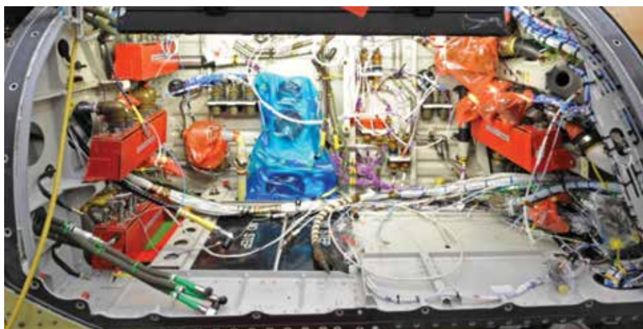
Figure 2: Typical Cable Installation in an Airframe
