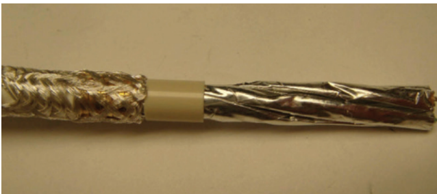
Figure 17: Sliding plastic bushing onto cable
