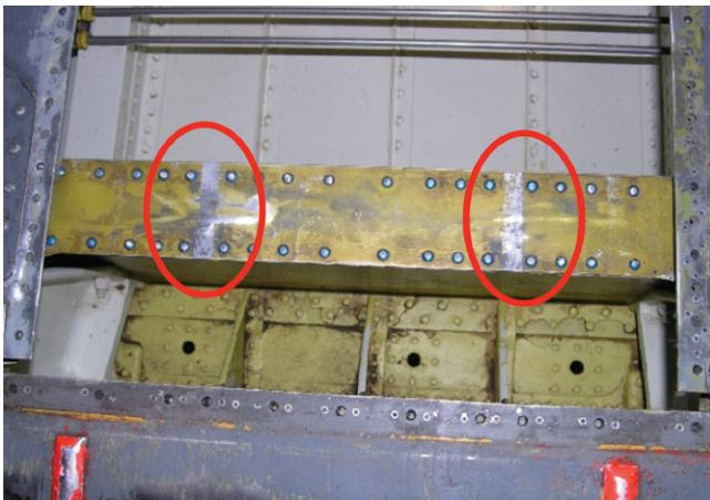
Figure 1: Chafing damage to the floor structure.
