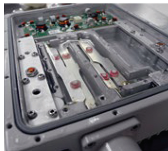
This combiner was returned from the field full of water
