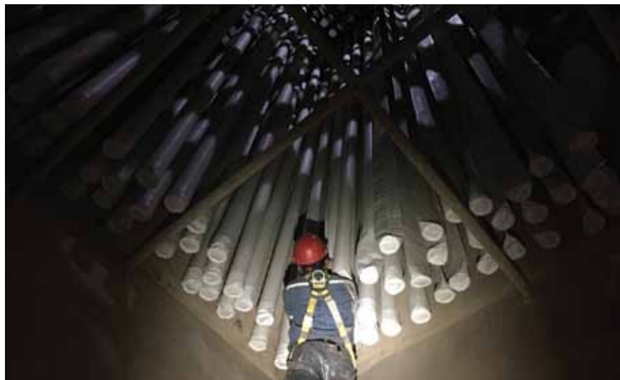
An example of how a cement plant's strategic investment in GORE® LOW DRAG Filter Bags has helped provide flexibility during economic extremes
