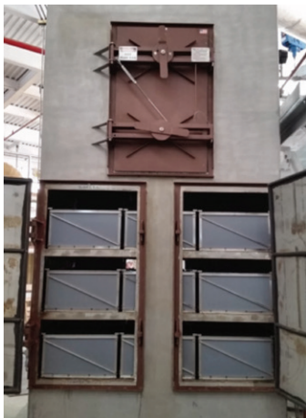
Stand-alone GMCS Installed After Scrubber at Sewage Sludge Incineration Facility (Photo Courtesy of EnviroCare International)
