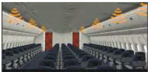
Figure 12 The leaky feeder antennas are mounted in the aircraft ceiling above the aisles.
