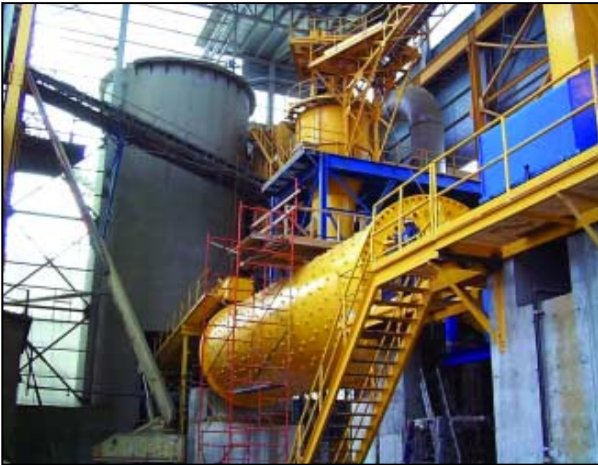
The 2250 kw cement mill before commissioning.
